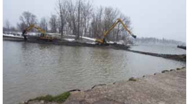
Dredging on April 6, 2016; looking south. Note gravel bar across the entire outlet.
