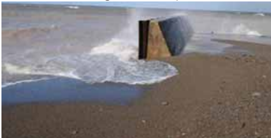
Gravel on pier, even at the toe of the concrete wall from the top of the wall; looking northeast
