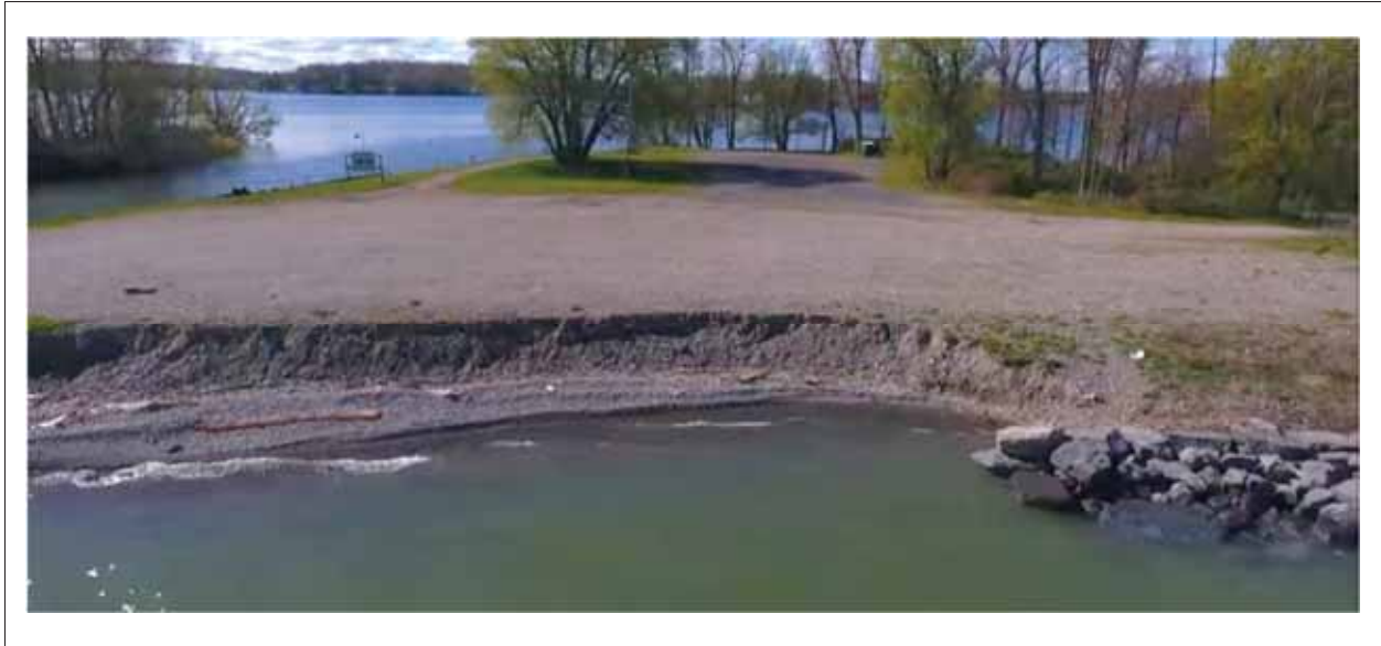
Figure 2.1-34 Wave-Induced Bank Erosion West of the Pier, May 10, 2017 (drone view)
